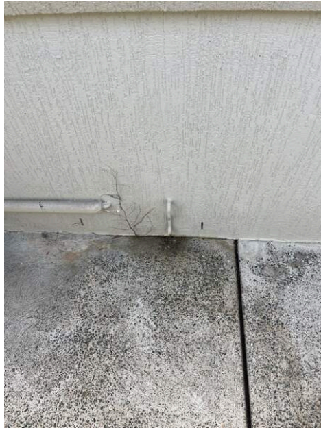
Photo Ref #3: The hot water system pressure relief valve should be redirected into a downpipe or away from the house as high moisture levels are conducive to timber pest activity.
