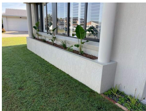
Photo Ref #4: The front garden beds abutting the external walls breach the termite barrier. Due to this a chemical
