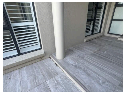
Photo Ref #5: The front entrance tiles breach the weep holes and the termite barrier. Due to this a chemical drill and
